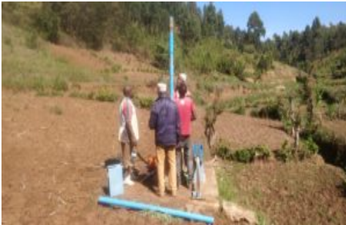
Water: (Dec21) we maintained the 11 BluePumps
